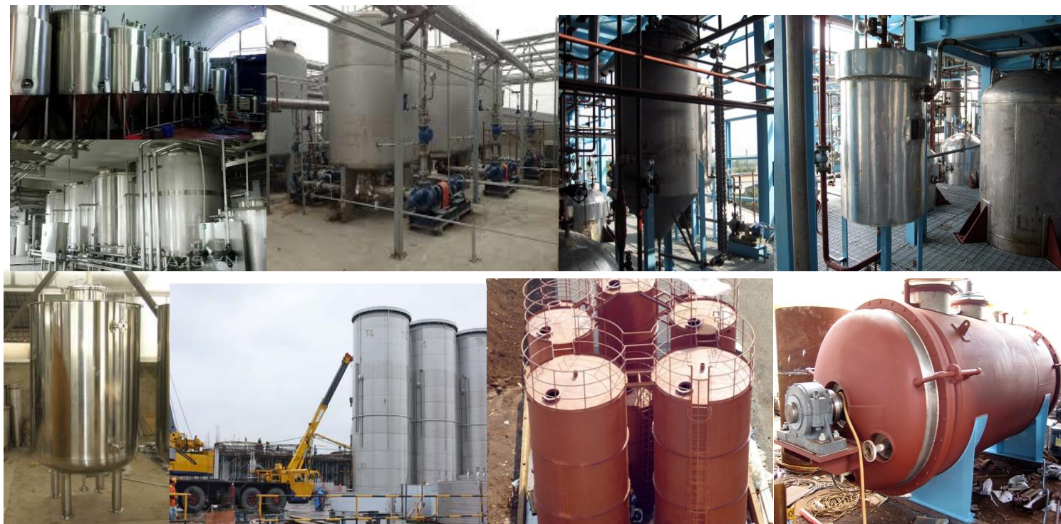
TANKS - INOX TANKS - COMPOSITE.
